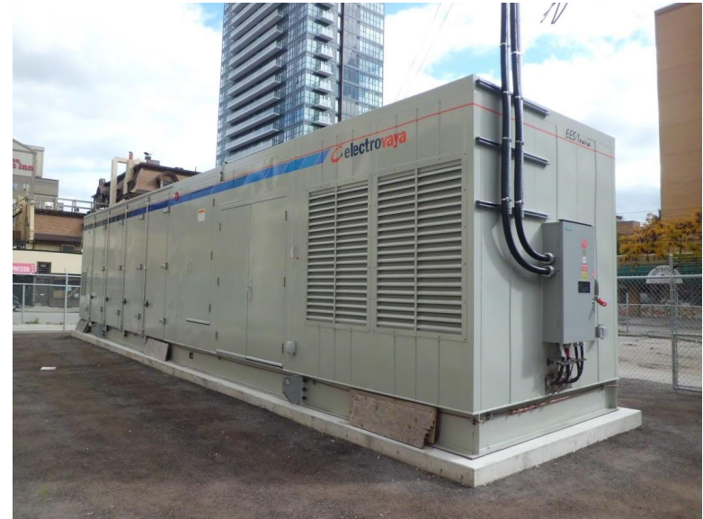
A grid scale Electrovaya energy storage system installed in Toronto, 2015
