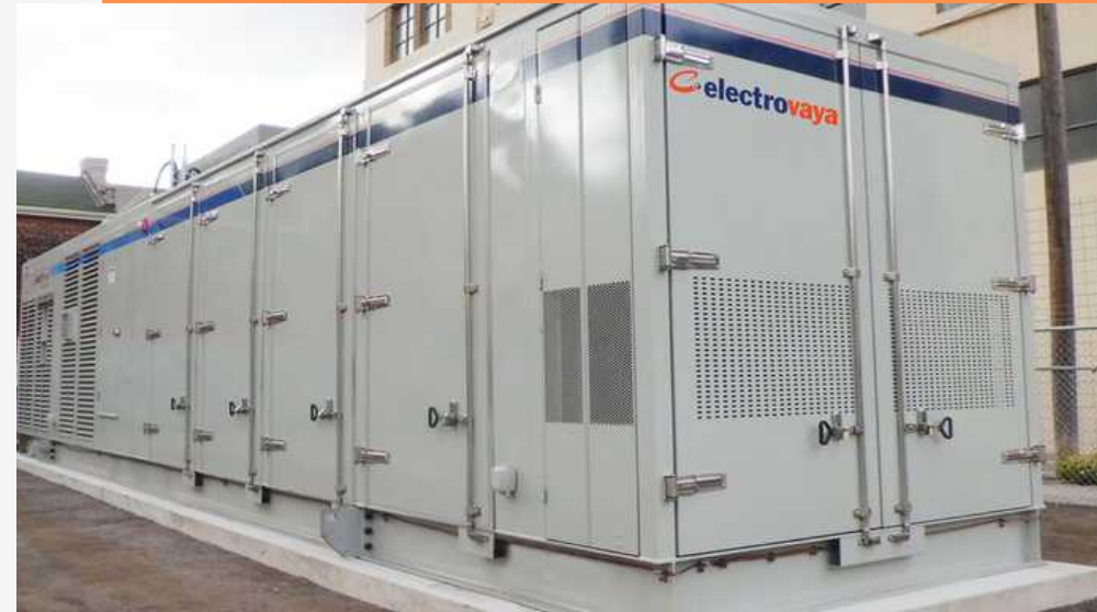
Electrovaya Battery Energy Storage System installed at Ryerson University in Downtown Toronto
