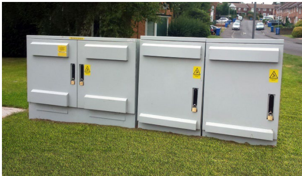
Energy Storage System installed in the UK with Scottish and Southern Energy
